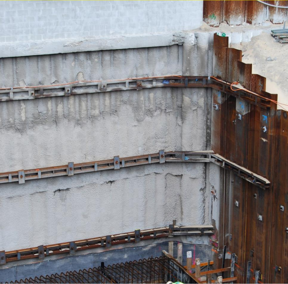
Above: CFA piles demonstrate their value in close proximity to neighbouring buildings and can combine with sheet piling.
